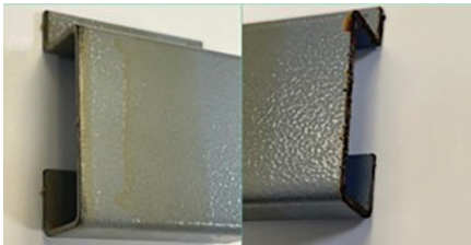
FIGURE 6 The uncoated cut edge shows obvious corrosion on the steel edge and under the FBE coating near the cut edge. Steel with FBE epoxy coating sustained corrosion from moisture laden with corrosive gases quickly when any coated surfaces are scratched or peeled away, exposing the bare steel surfaces.
