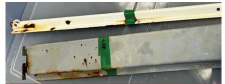
FIGURE 5 Steel bars coated with epoxy coatings were partially coated with field applicable 100% PVDF topcoat (~50µm thickness). The portion protected by epoxy coatings only when exposed to salt-water (water with dissolved corrosive ions) suffered extensive corrosion in 65 days under the accelerated conditions of 60°C-5% saline solution. By comparison, epoxy-coated steel when top-coated with field-applicable PVDF coating showed no sign of corrosion. The accelerated conditions are roughly equivalent to two to three years of ambient temperature seawater submersion conditions.
